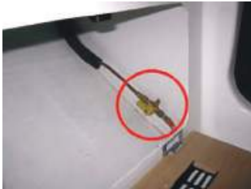
Gas supply valve
