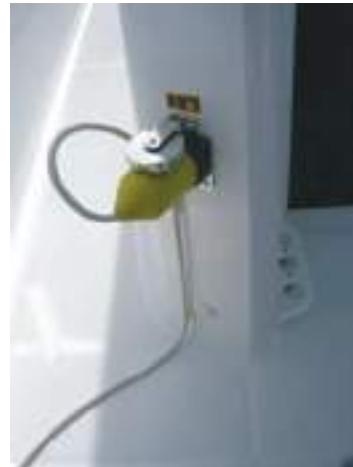
Shore power socket Ref 1
