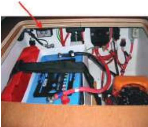
Operation relay Location: Forward cabin
