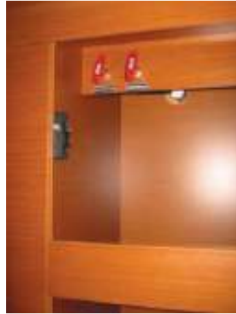
Remote shut-off pull handle Location: Aft cabin
