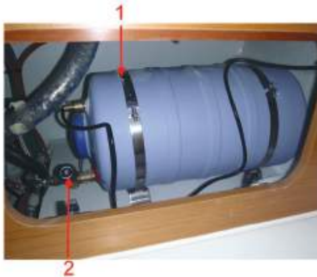
Water heater Access: Aft cabin
