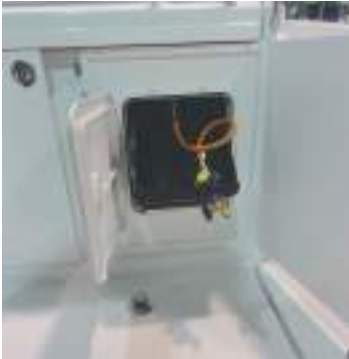
Gas cylinder locker
