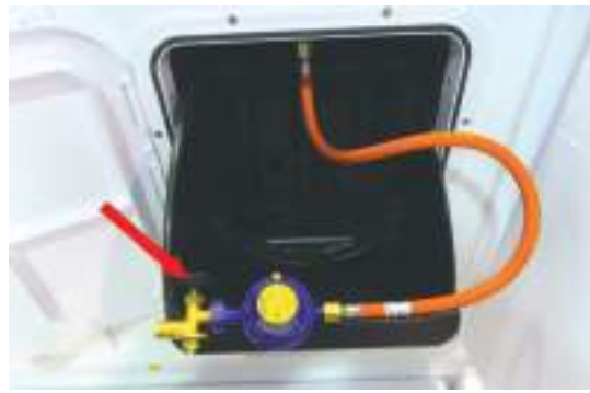
Supply valve - Gas
