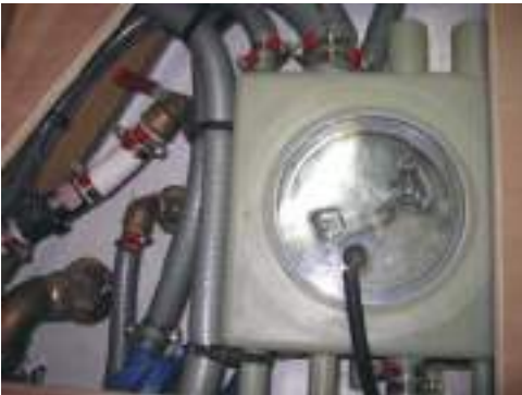
Collector - Waste water
