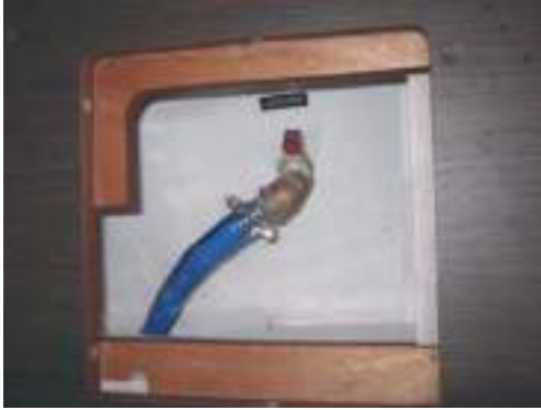
Sea water intake Location: Skipper's cabin
