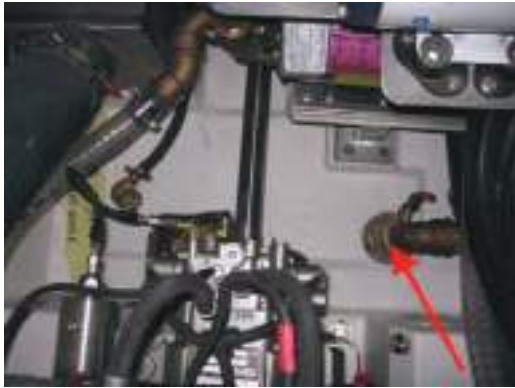
Sea water intake
