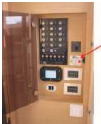
Location: Electrical panel
