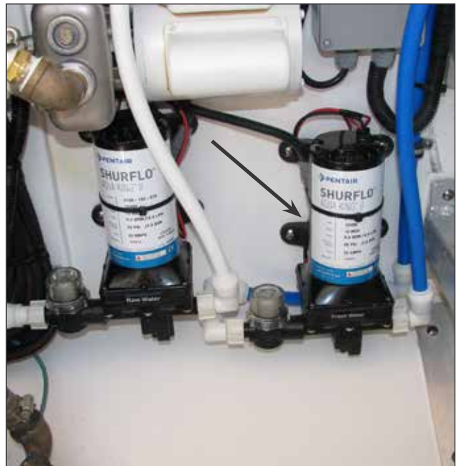
Fresh Water Pump & Strainer
