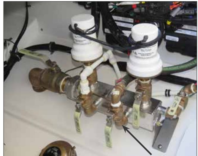
Air Conditioner Pump Supply Valve
