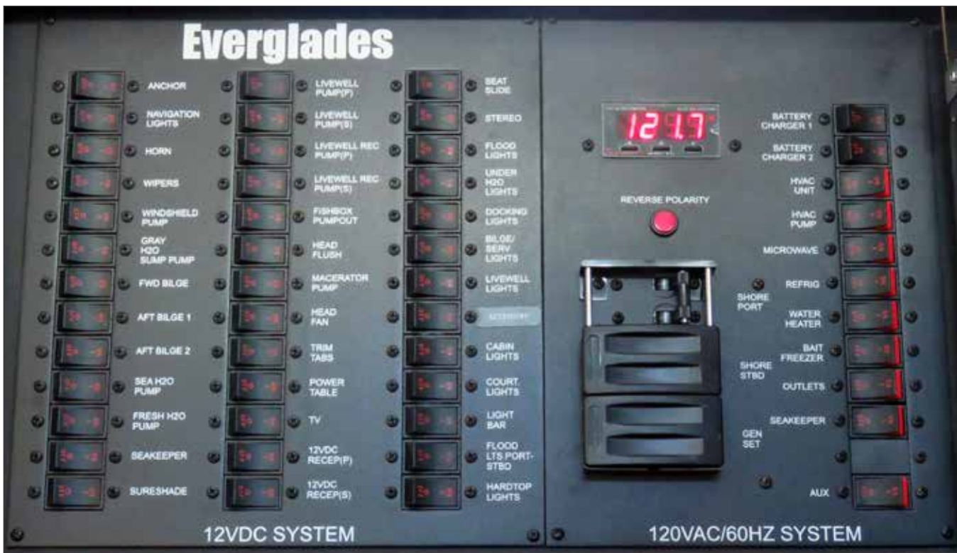
Cabin DC/AC Panel
