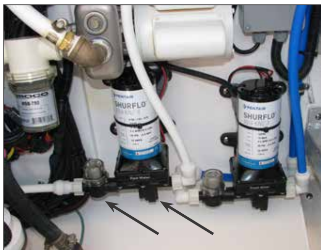
Raw Water Pressure Pump & Sea Strainer
