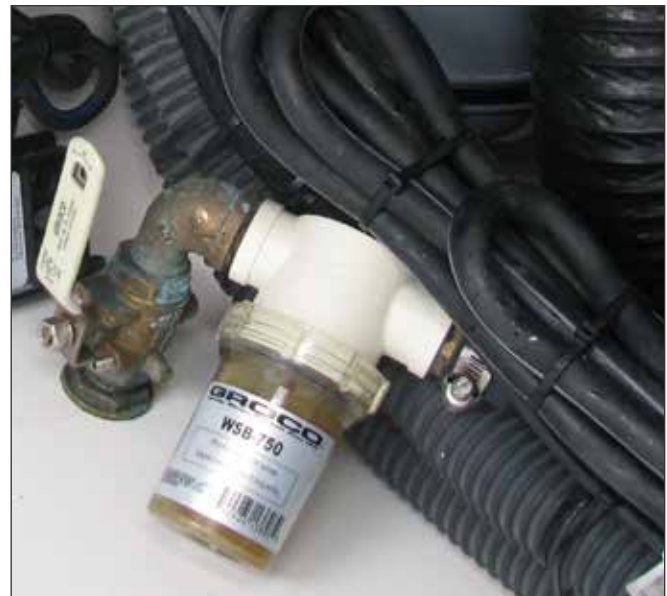
Generator Sea Strainer & Seacock
