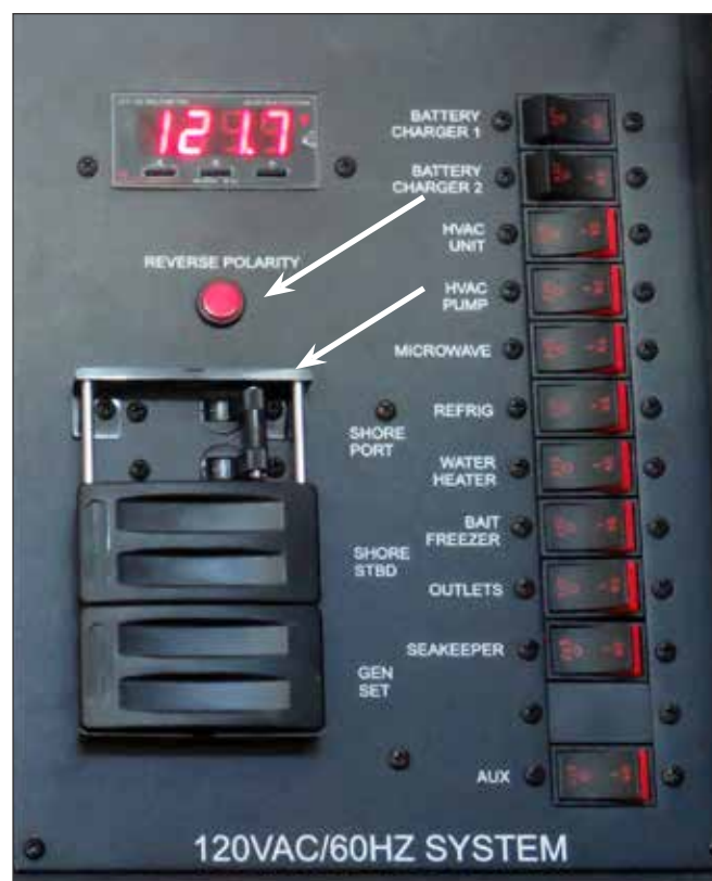
Reversed Polarity Light & Shore PWR/Generator Main Breakers
