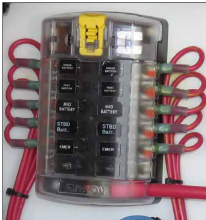
Remote Battery Switch Fuse Panel
