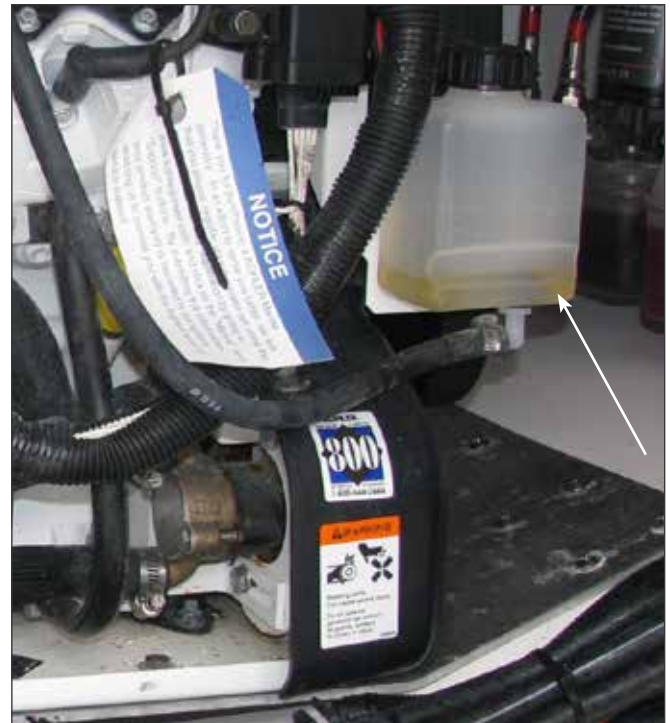
Typical Generator Coolant Recovery Tank
