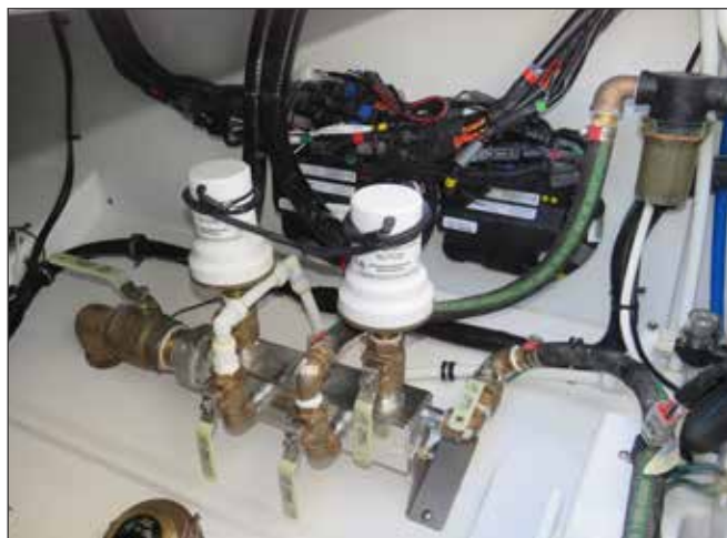
Raw Water Manifold, Port & Starboard Livewell Pumps, Raw Water Pump Connection, HVAC Pump Connection & Ball Valves
