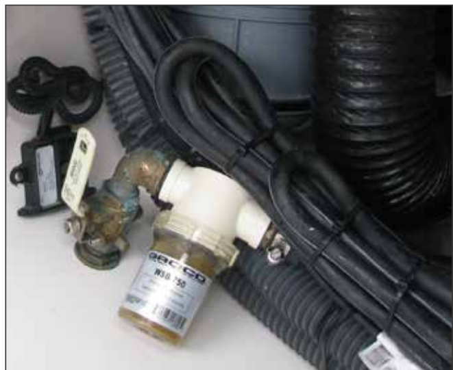
Typical Generator Raw Water Seacock & Strainer
