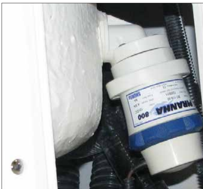
Typical Livewell Recirculation Pump
