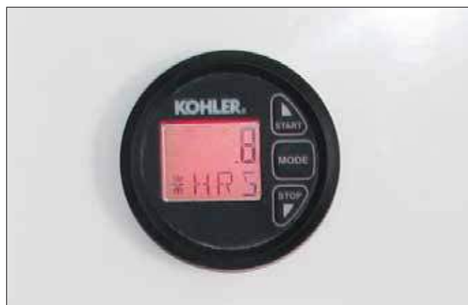
Cabin Generator Control Switch & Monitor
