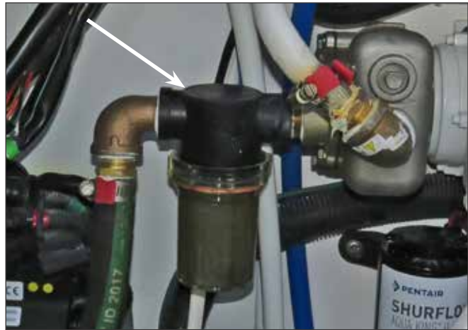
HVAC Pump Sea Strainer
