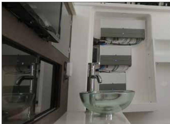
Starboard Electronic Module Mounting Area
