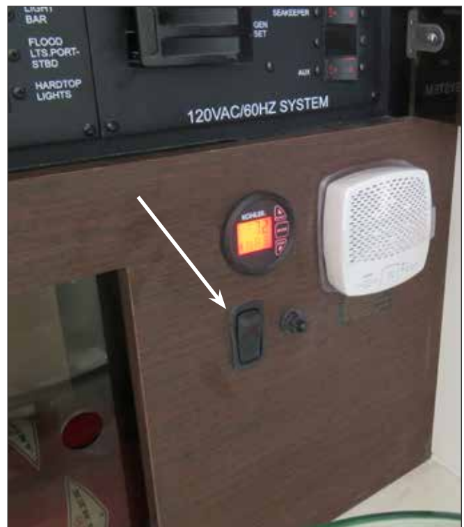
Cabin Bilge Blower Switch
