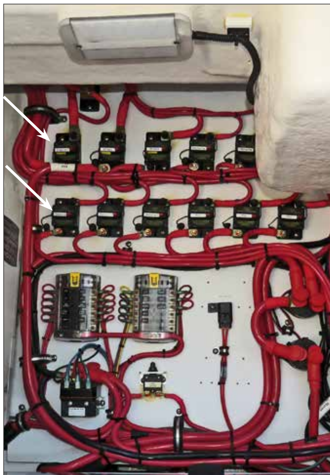
Heavy Duty Main Circuit Breakers
