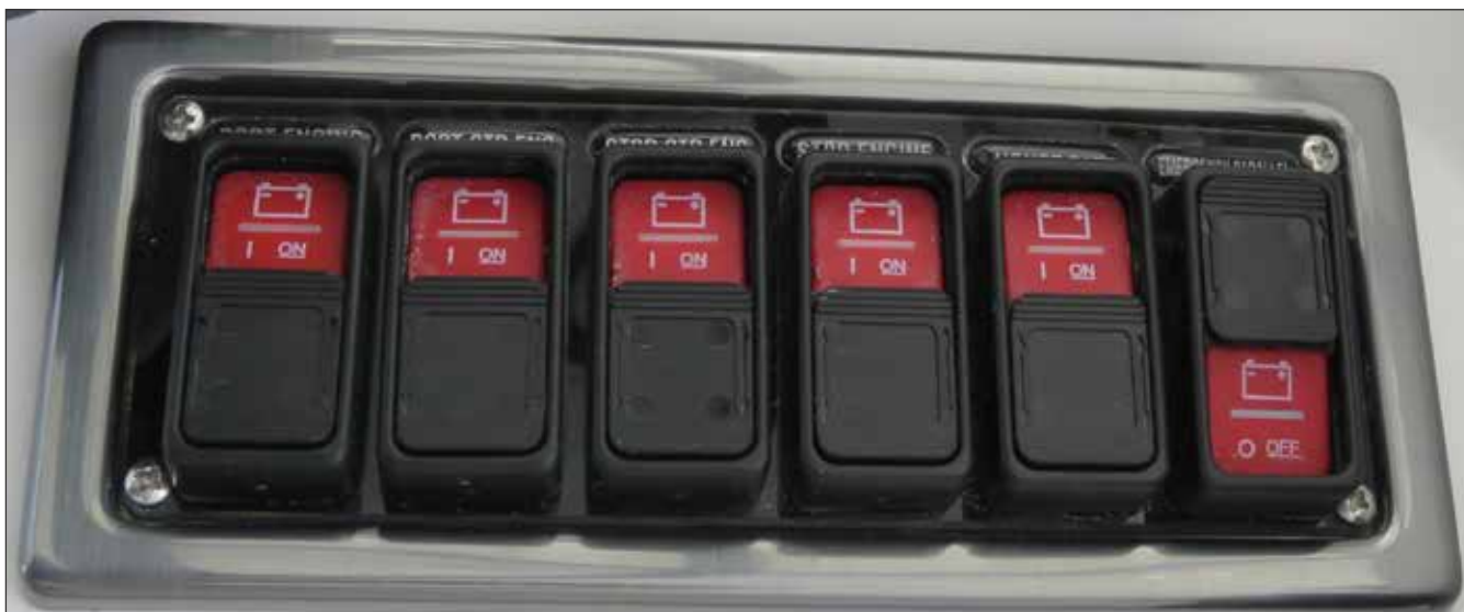
Battery Switch Panel at Helm
