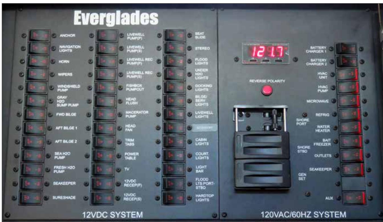
Cabin DC/AC Panel
