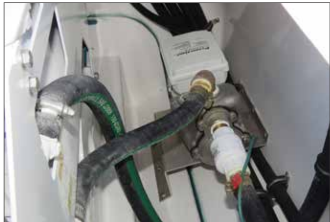
Typical SeaKeeper Seawater Pump
