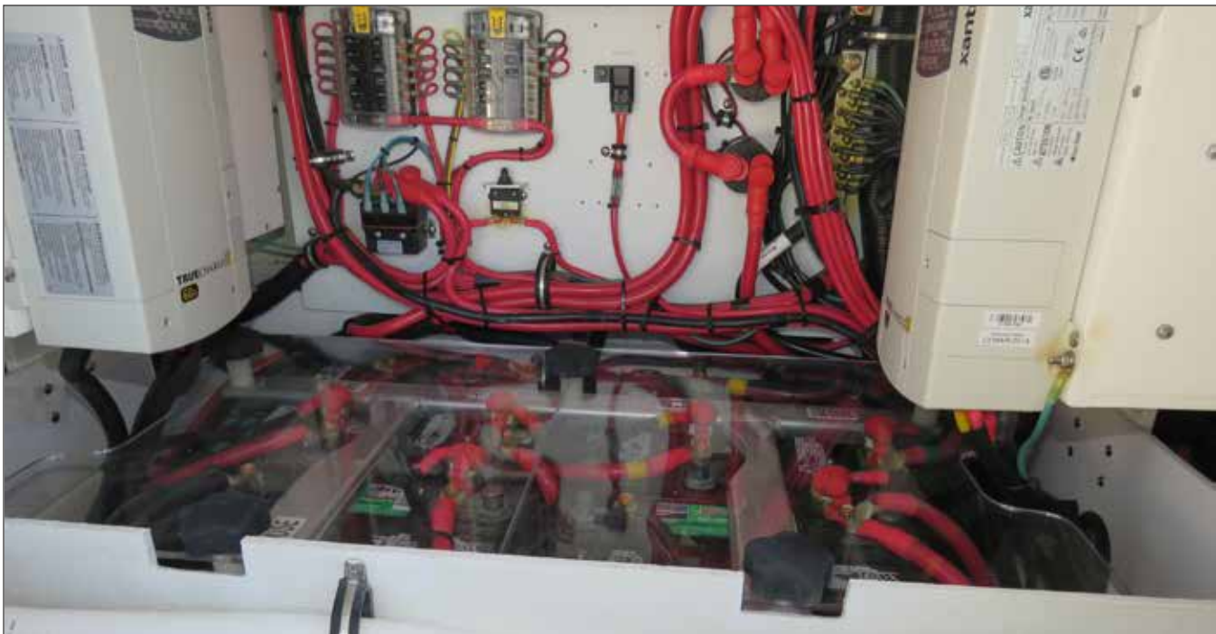
Batteries In Electrical Systems Compartment
