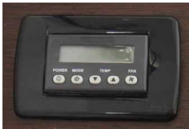
Air Conditioner Control Panel
