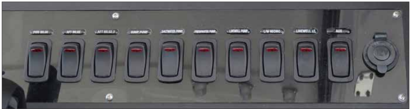
Starboard Helm Accessory Switch Panel
