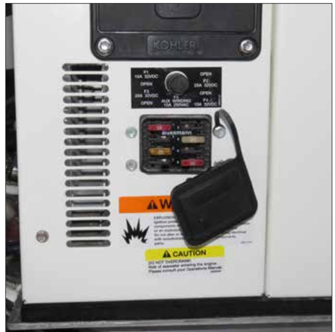
Typical Generator Fuse Panel
