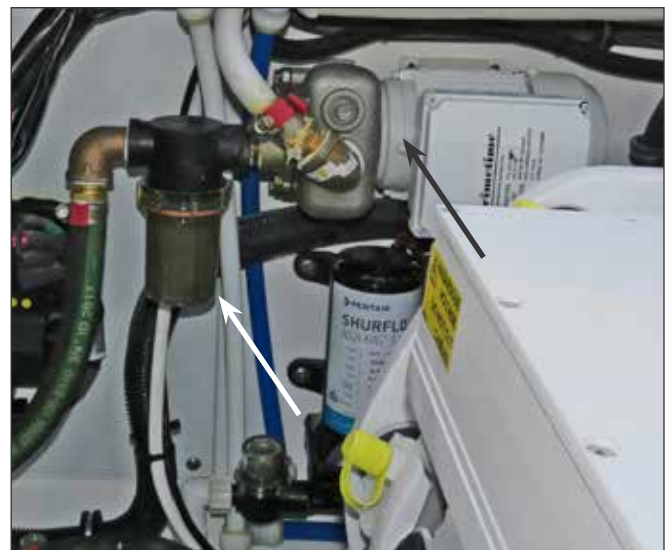
Air Conditioner Seawater Pump & Strainer
