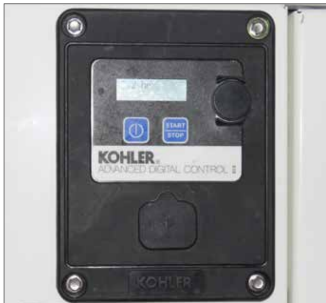
Generator Onboard Control Switch & Engine Monitor,
