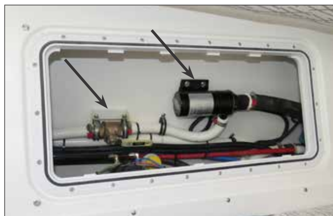
Overboard Macerator Pump & Thru-Hull Valve
