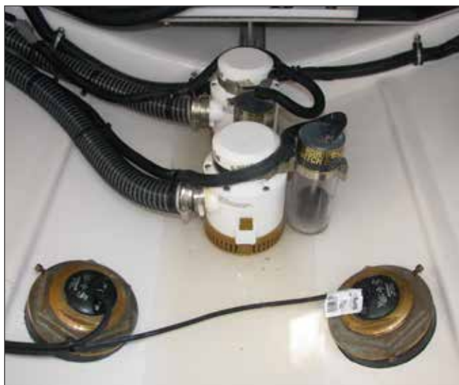
typical Stern Bilge Pumps & Automatic Switches
