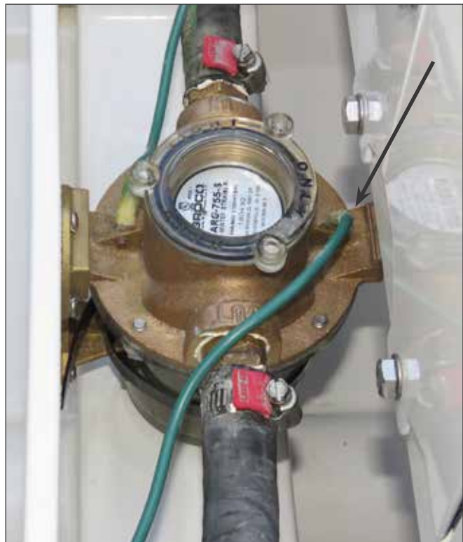
Typical Sea Strainer Bonding Wire
