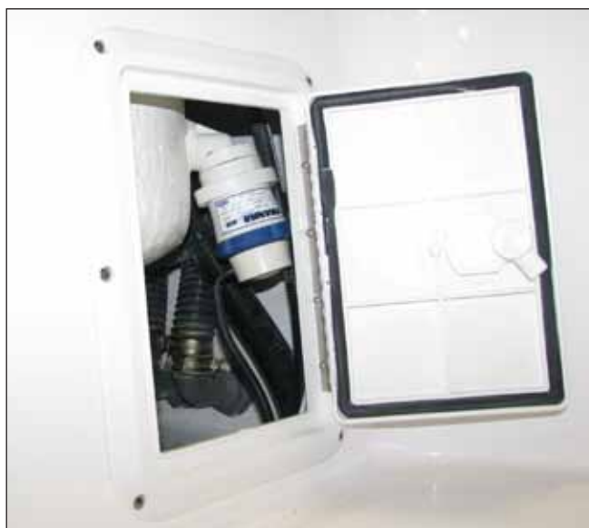
Livewell Recirculation Pump
