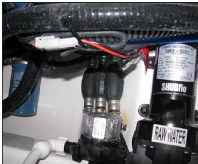
Primer Bulbs Near Fuel Filters
