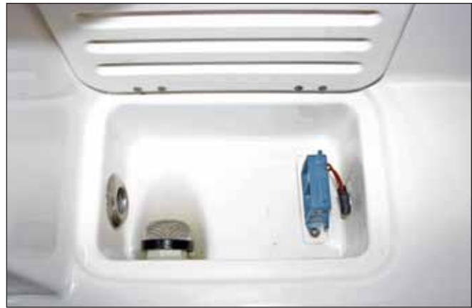
Head and Shower Sump System
