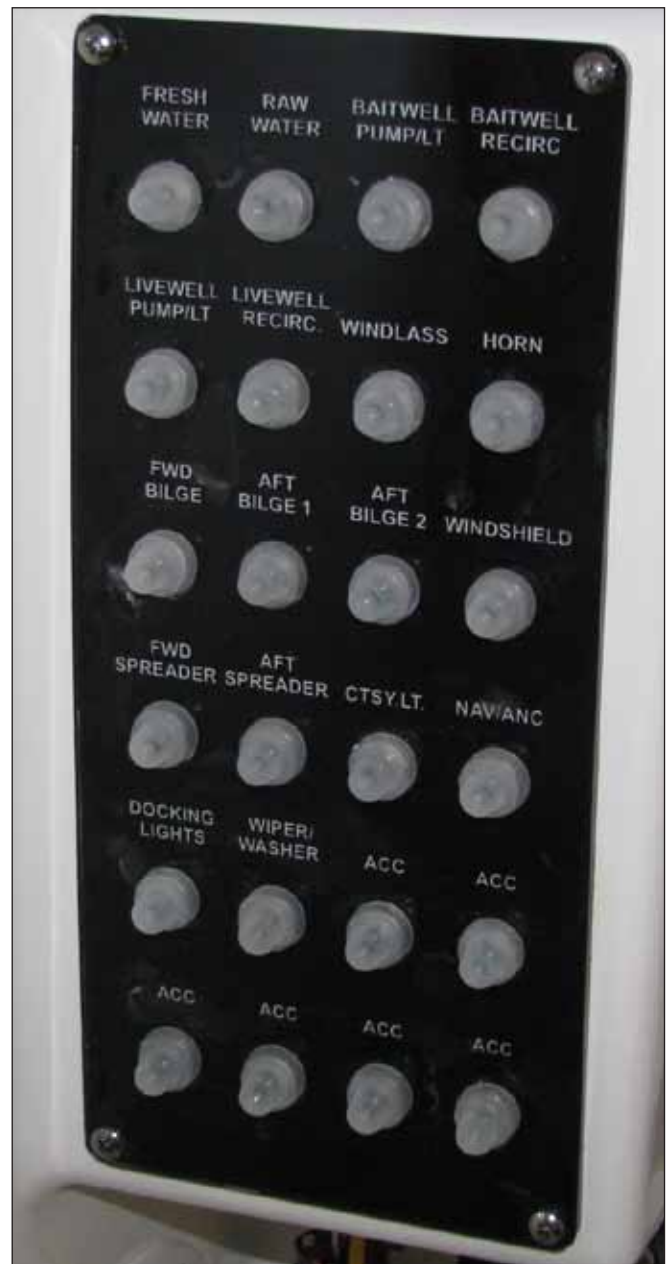
Head Compartment Circuit Breaker Panel
