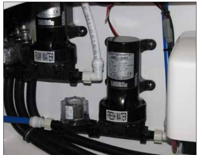
Fresh Water Pump and Strainer
