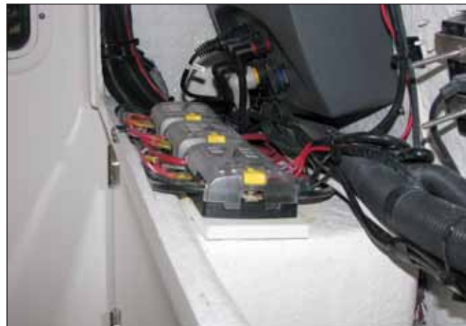
Fuse Panels Behind Helm
