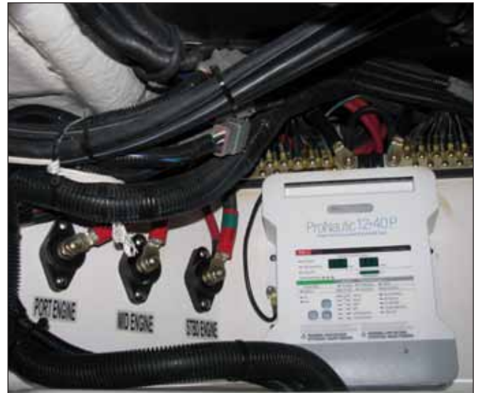
Typical Battery Charger in Systems Compartment
