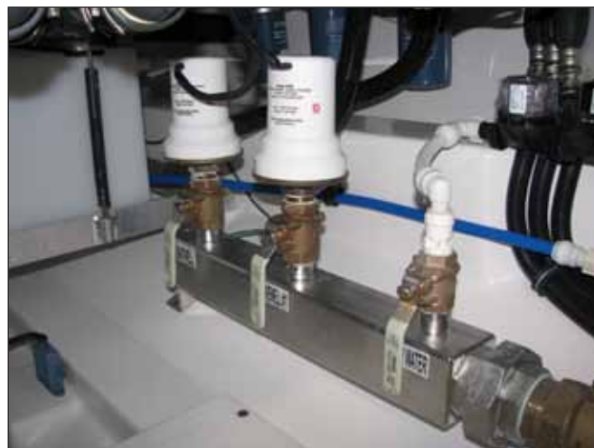
Raw Water Manifold, Livewell Pump, Baitwell Pump, Raw Water Supply Pump Connection and Ball Valves
