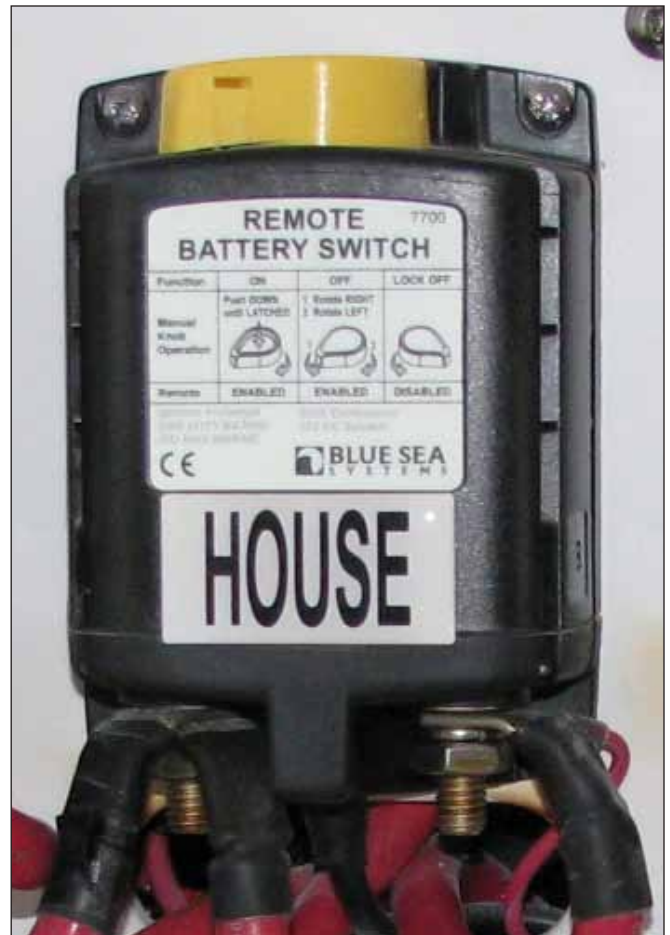
Typical Remote Battery Switch
