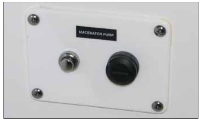
Typical Waste Discharge and Lockout Switches
