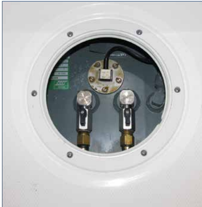
Fuel Withdrawal Valves & Tank Sending Unit
