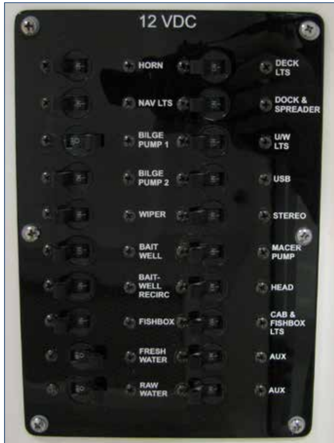
Accessory Circuit Breaker Panel In Head Compartment
