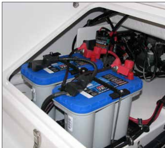
Typical AGM Batteries
