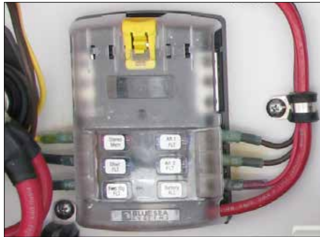
Typical Helm Accessory/Electronics Fuse Panel
