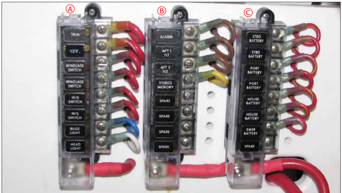
Accessory & Continuous Power Fuse Panels In Aft Systems Compartment A) Accessory Fuse Panel B) Continuous Power Fuse Panel C) Remote Battery Switch Fuse Panel
