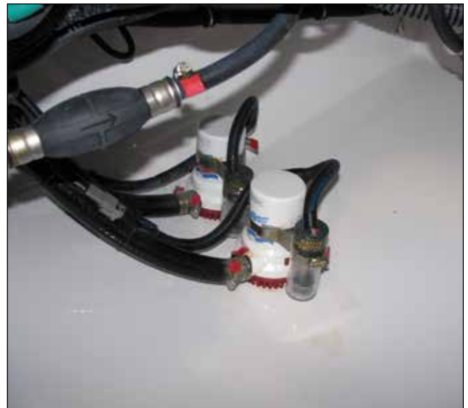
Aft Bilge Pumps & Automatic Switches
