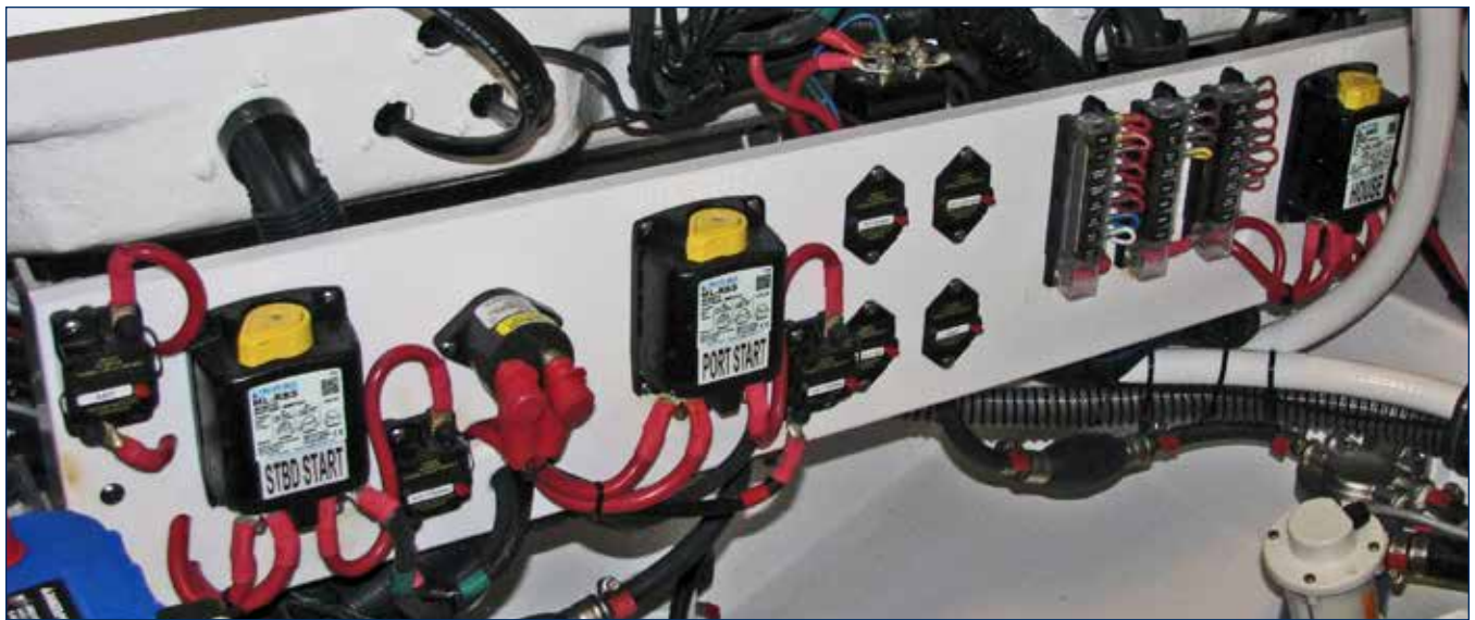
Battery Switch Panel In Aft Systems Compartment
