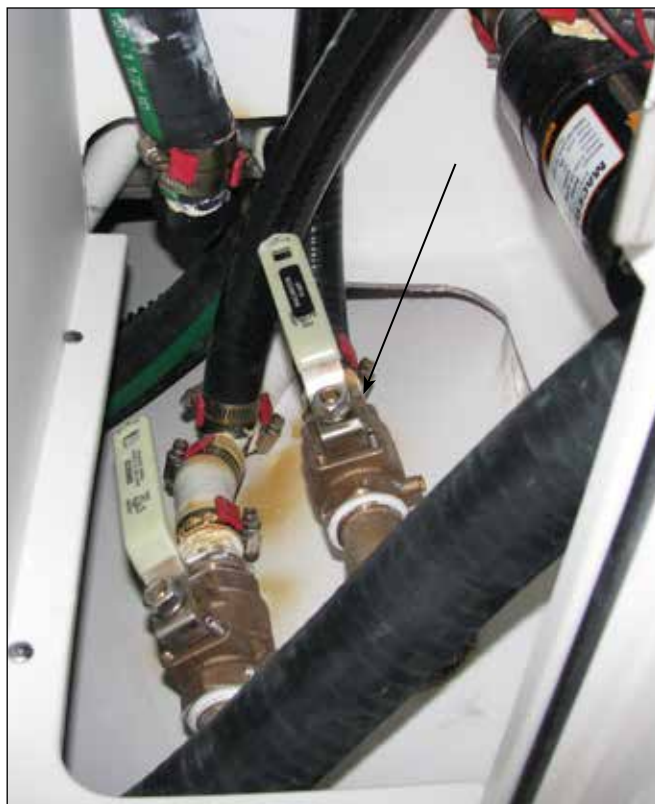
Overboard Discharge Thru-Hull Valve
