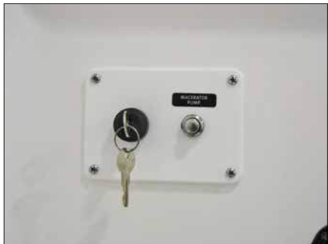
Waste System Pump Out Switch Panel
