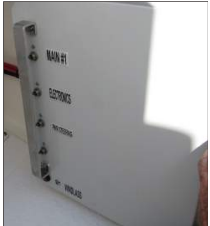
325 Center Console Main Circuit Breakers
