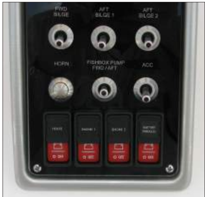
Remote Battery Switches in OFF Position
