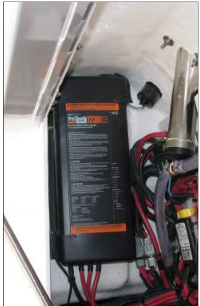
Typical Battery Charger
