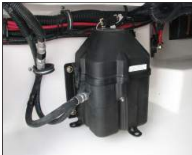
Power Steering Unit in Stern Bilge
