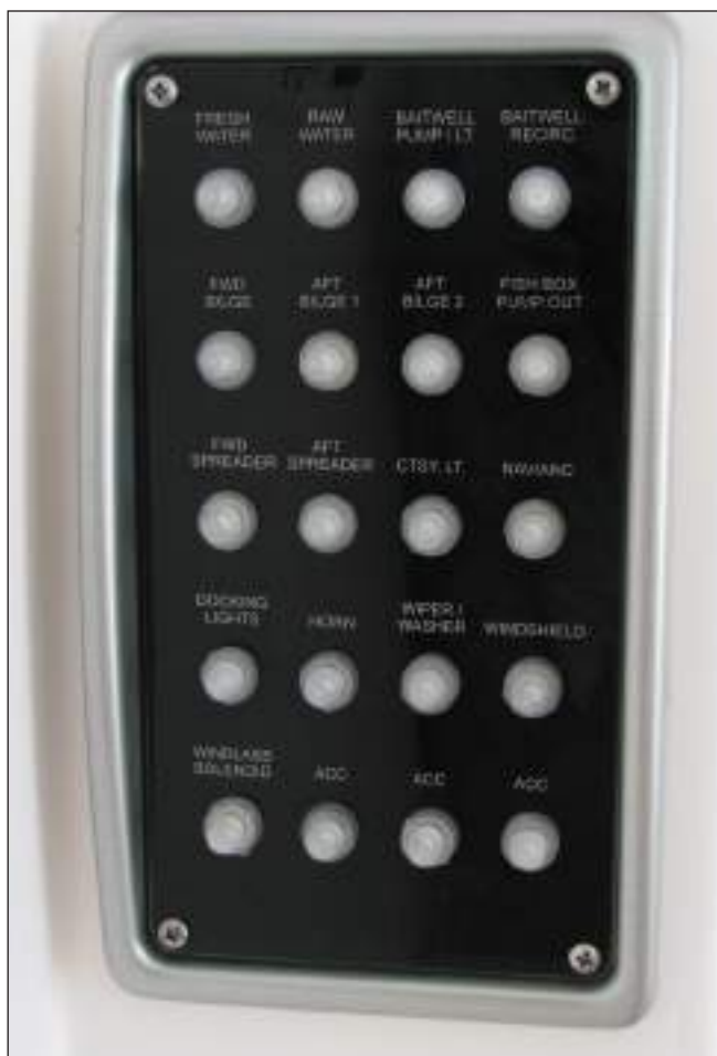
Head Compartment DC Circuit Breaker Panel
