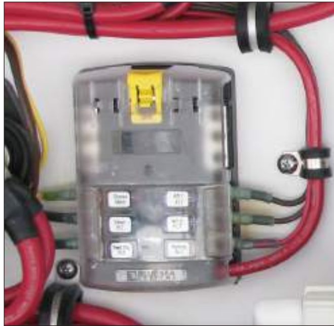
Continuous Power Fuse Panel
