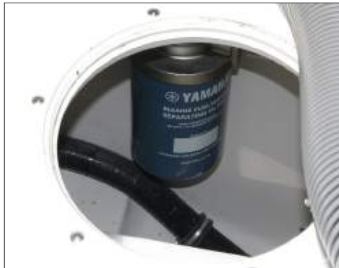
275/295 Center Console Fuel Filters Below Splashwell
