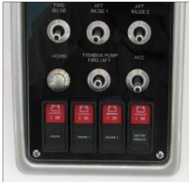
Remote Battery Switches in ON Position
