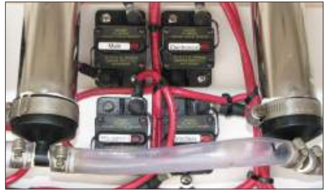
255/275/295 Center Console Main Circuit Breakers
