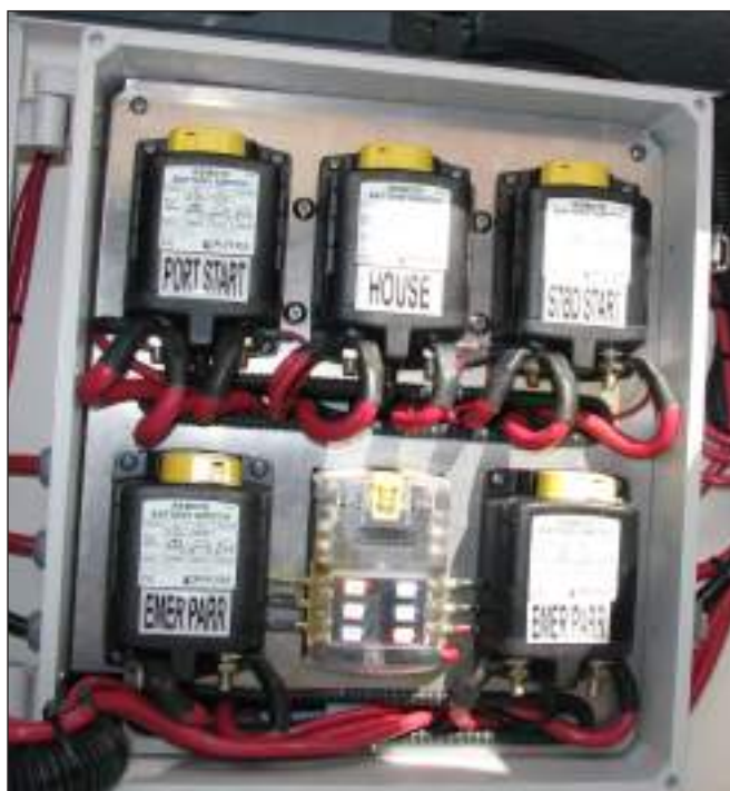
325 Center Console Battery and Emergency Parallel Switches
