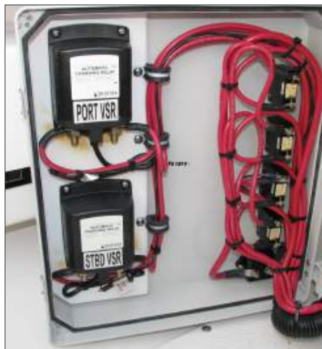
325 Center Console Voltage Sensitive Relays
