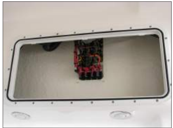
Helm Access Panel in Head Compartment
