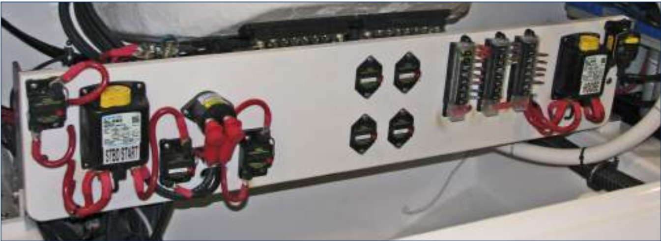
Battery Switch Panel In Aft Systems Compartment
