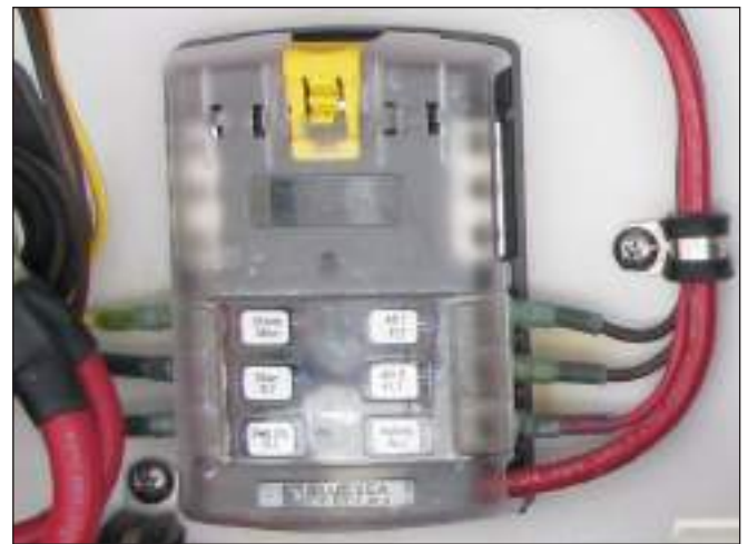
Typical Helm Accessory/Electronics Fuse Panel
