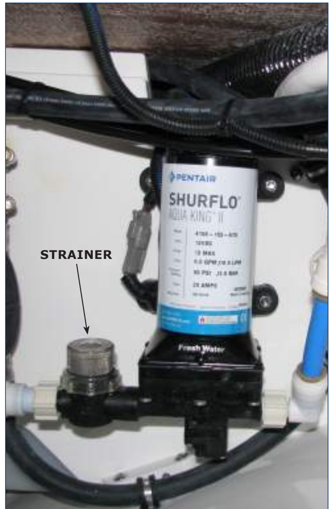
Raw Water Pressure Pump & Sea Strainer
