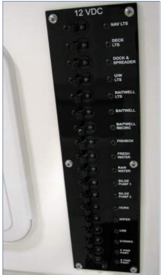
Accessory Circuit Breaker Panel In Head Compartment
