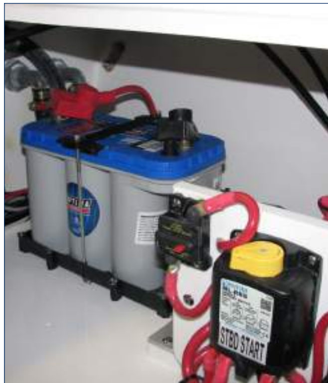
Typical AGM Battery
