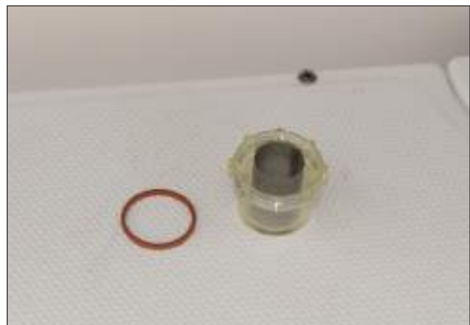
Typical Fresh Water Pump Strainer Removed for Cleaning
