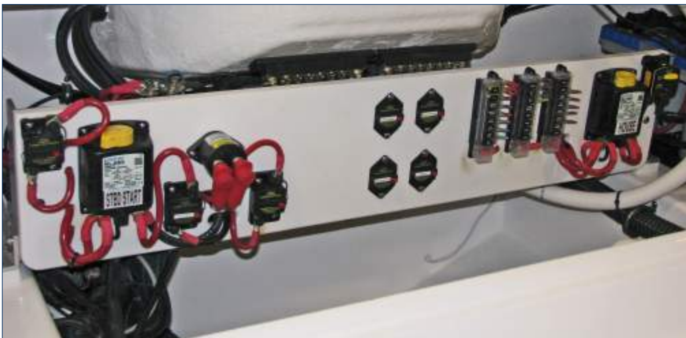
Battery Switches, Fuse Panels & Main Circuit Breakers
