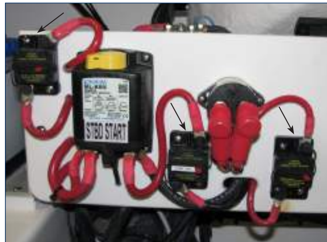
AMP & Engine Main Circuit Breakers
