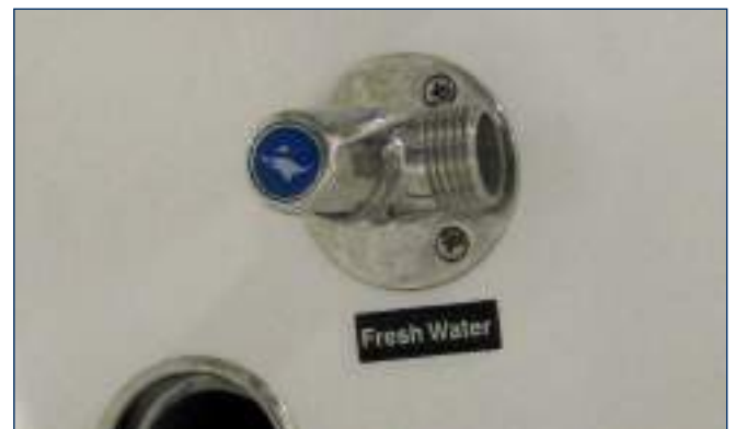
Fresh Water Washdown Hose Connection
