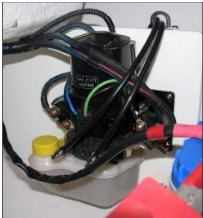
Hydraulic Pump System for Windshield In Aft Systems Compartment
