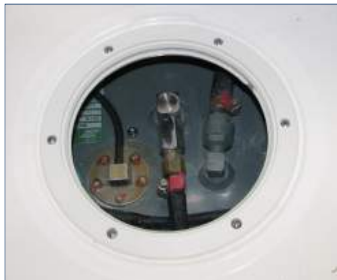
Fuel Withdrawal Valves & Tank Sending Unit
