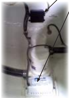
Typical Aft Bilge Pump - 54 Voyager Bilge Similar
