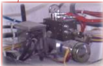
Hydraulic Pump (Engine Rm. Bilge Area)
