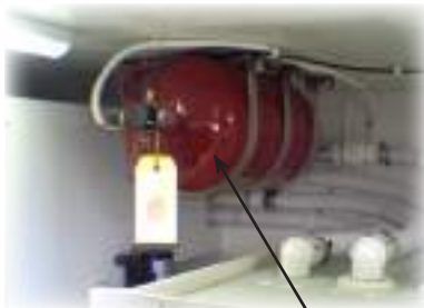
Typical Fire Suppression Tank (54 V Similar)
