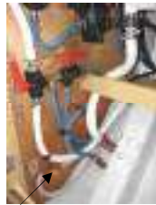
Location of cock below sink
