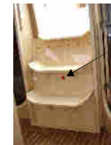
Engine compartment fire-extinguisher hose hole Location between main companionway steps
